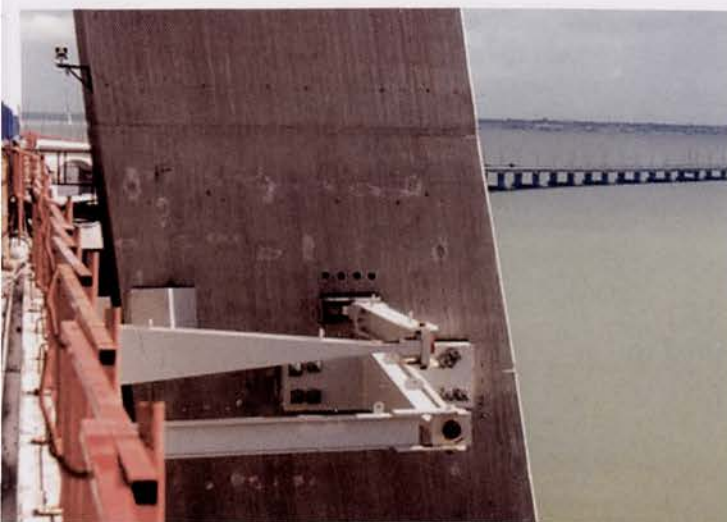
Amortecedores entre o tabuleiro e as torres Dampers between the deck and the towers
