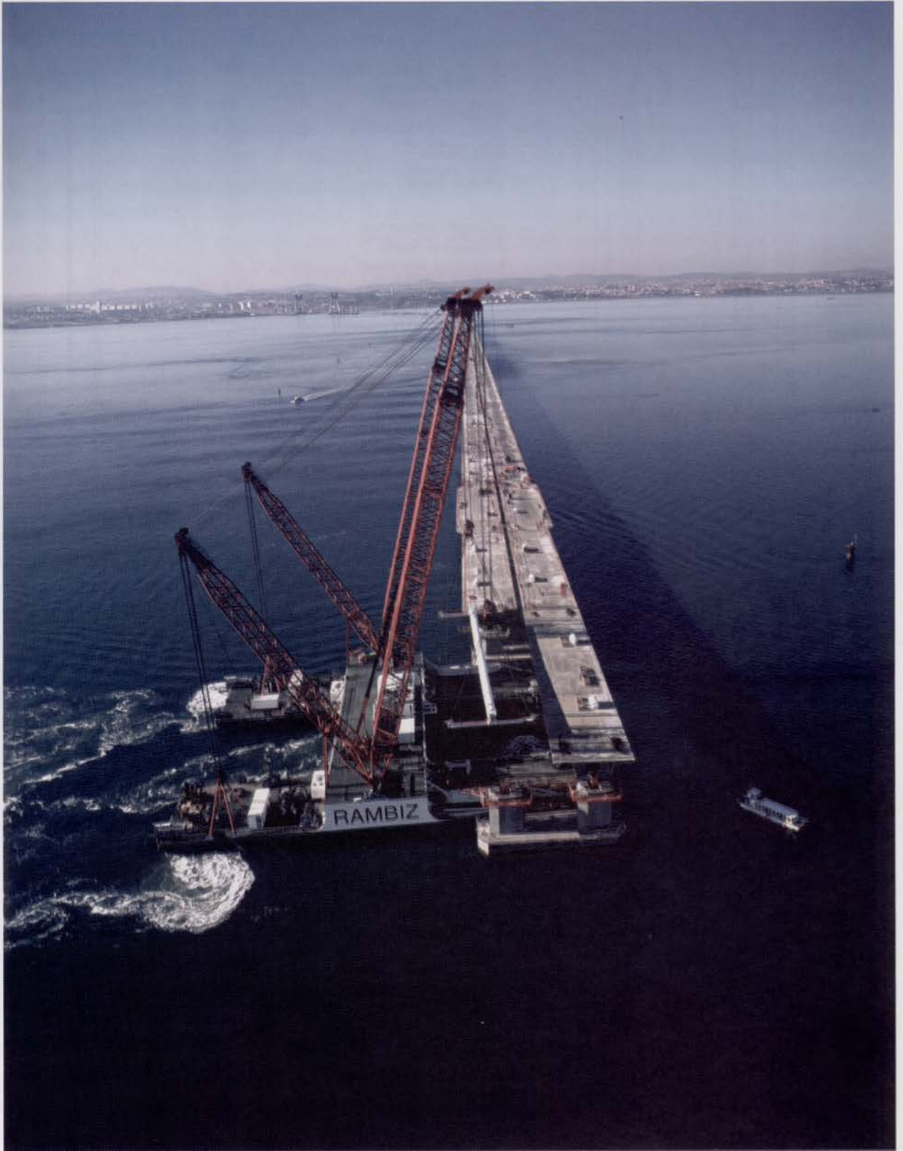
Viaduto central, montagem de viga com 78 m, com a grua Rambiz Central viaduct, installing 78m beam with the Rambiz crane ship
